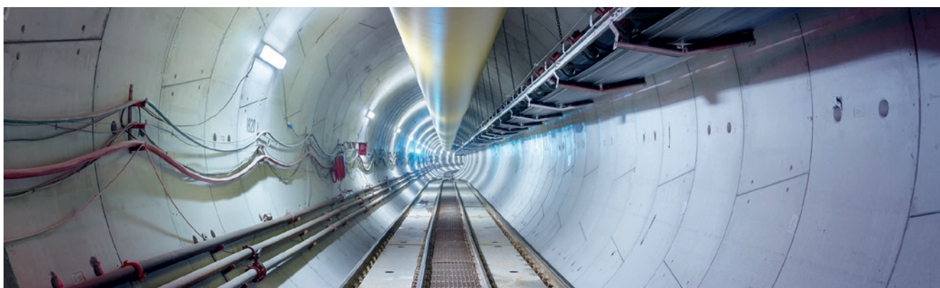
SDS at STEP Tunnel Contract (T-02/T-03) Deep Tunnel Sewer in Abu Dhabi
